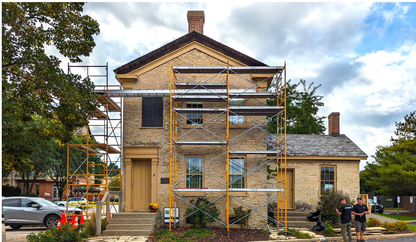
First part of deteriorated trim removed at the William Beith House, September 25, 2023
